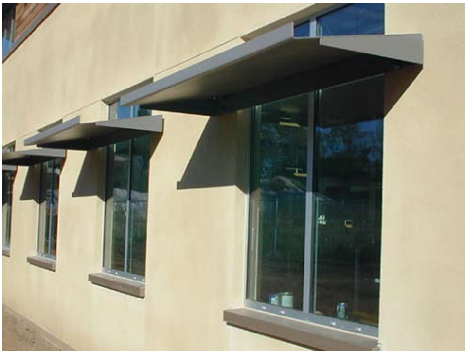
This photo shows the sun shades and lightshelves.
