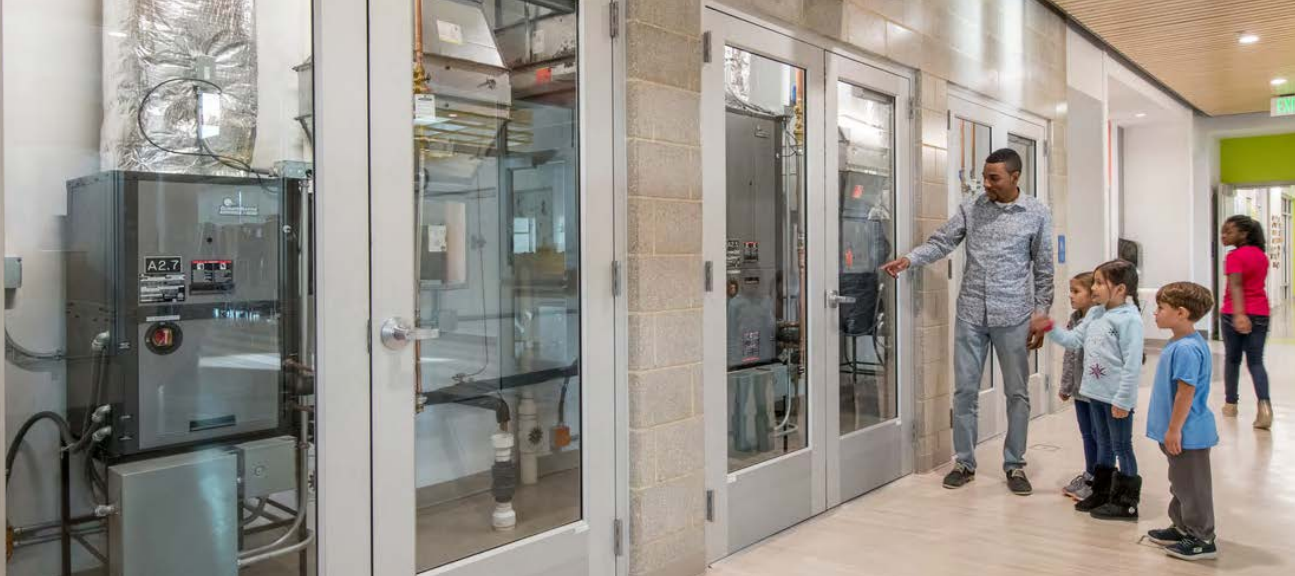
Martice Tucker , a former intern and now co-worker, explains geothermal heat pump equipment to students through glass doors that he helped to design in the corridor at Moncure ES under Amy's sustainability education leadership.
