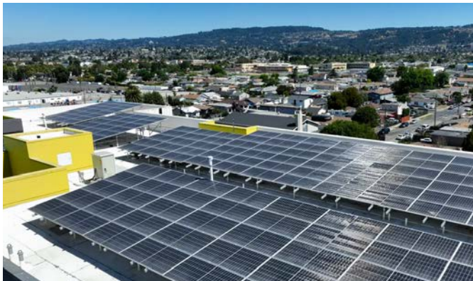
On-site solar produces all of the energy required for house loads. Photo Credit: Jeff Durkin
